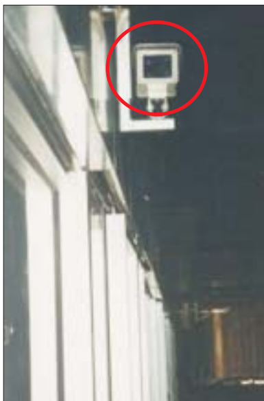
Fig. 4 • Kuala Lumpur Aiport terminal - ERL door control signals are transmitted from the train to the platform
